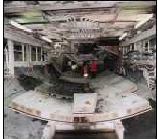
Rear view showing the pre-formed, steel-reinforced tubbings that will form the tunnel lining
